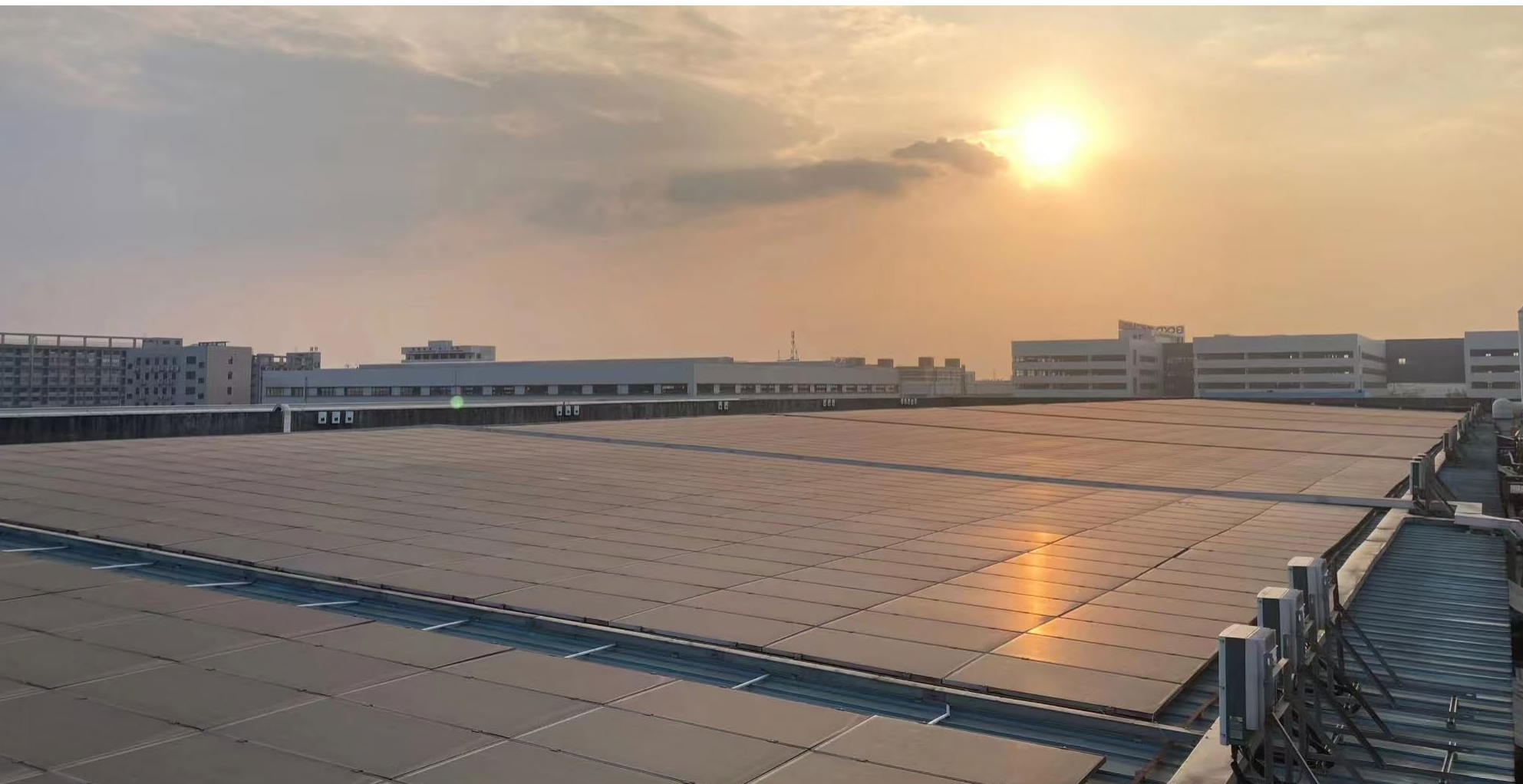
Foshan Base PV Generation Project on Rooftops
