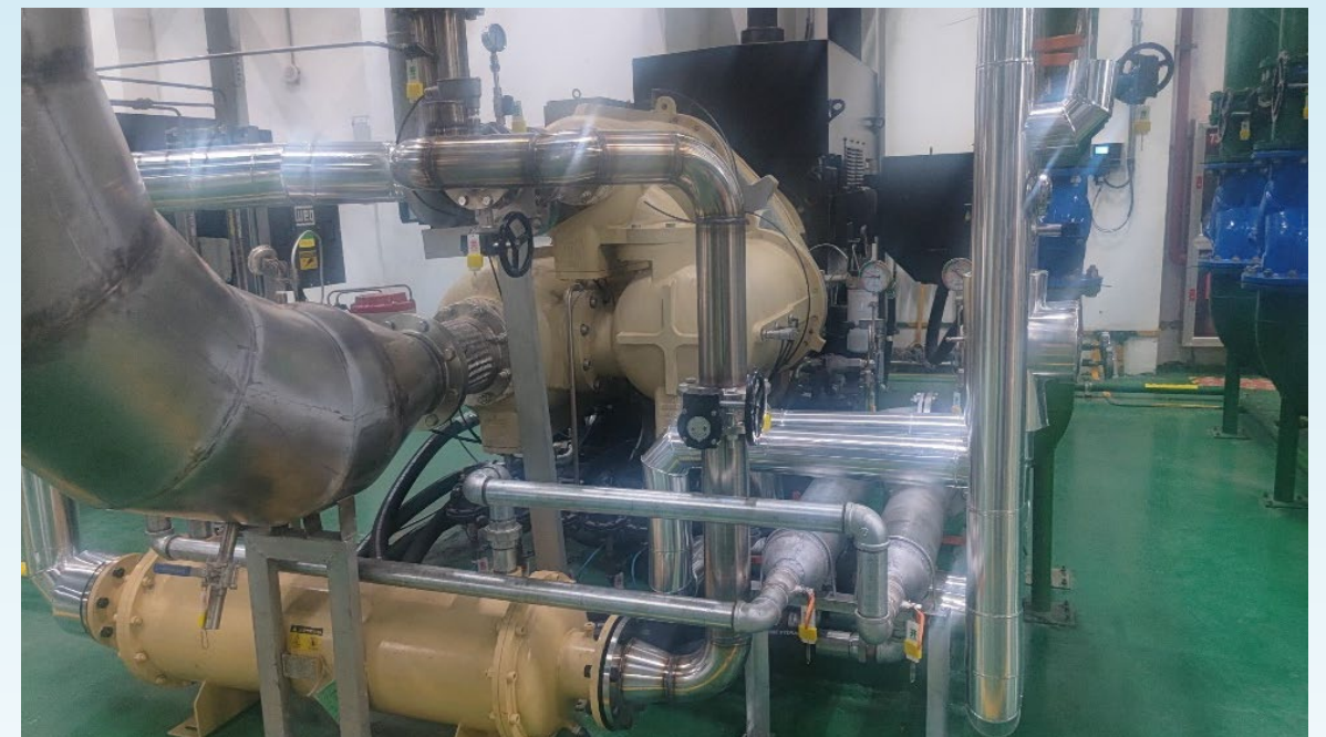
Heat Transport Pipelines
