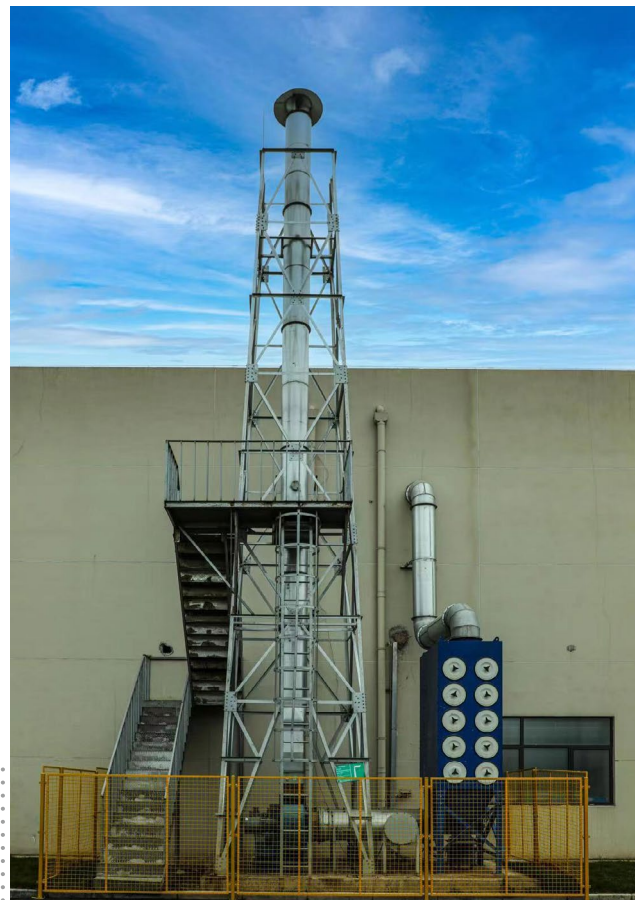
Waste Gas Treatment Facilities
