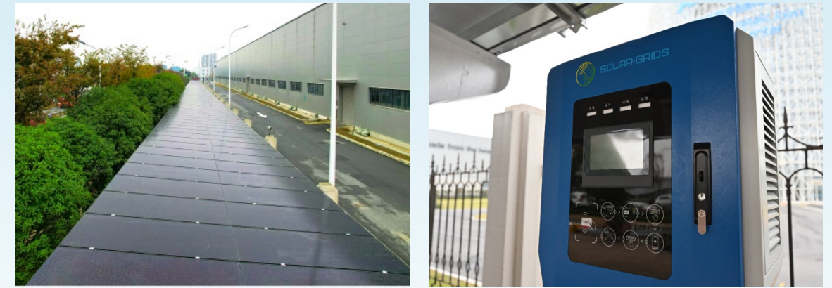
PV Car Parking Shed
