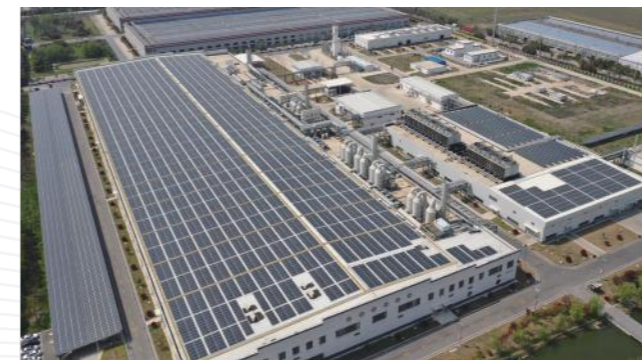
Jianhu County Distributed PV Project 5.5MWp
