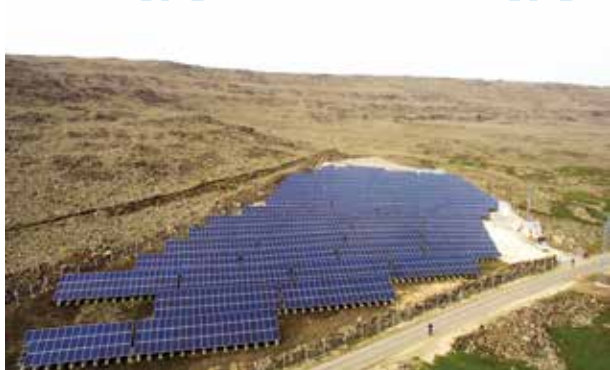
GAZİANTEP ŞEHİTKAMİL 1.3 MWp - 2016
