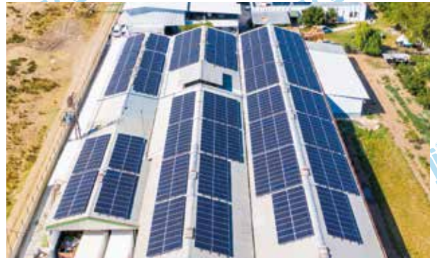
BURSA YENİŞEHİR 315 kWp - 2021
