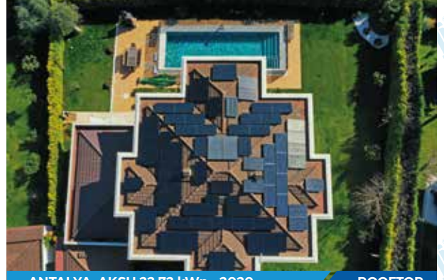
ANTALYA AKSU 22.72 kWp - 2020 ROOFTOP
