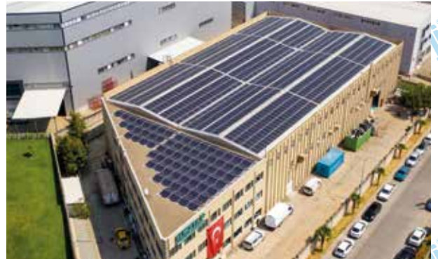
BURSA OSMANGAZI 342 kWp - 2019
