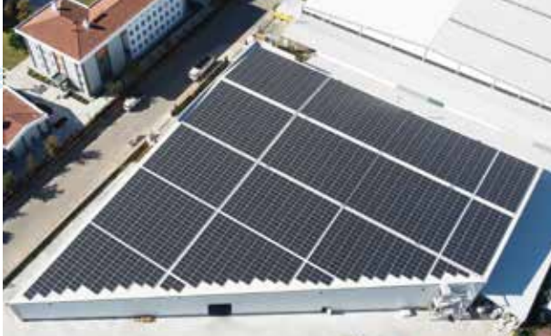
ANTALYA OSB 800 kWp - 2021
