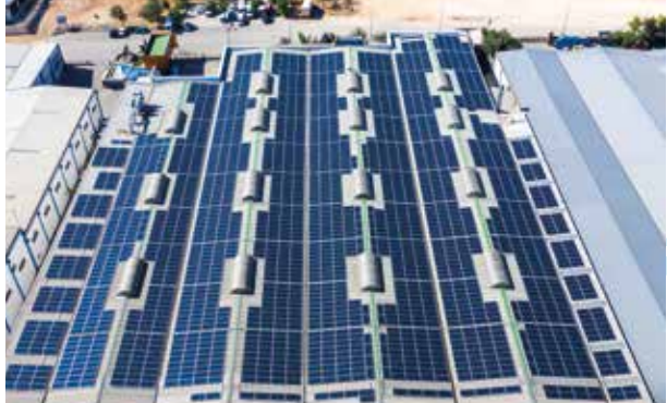
GAZİANTEP ŞEHİTKAMİL 938 kWp - 2021
