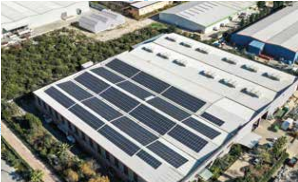
ANTALYA OSB 400 kWp - 2015
