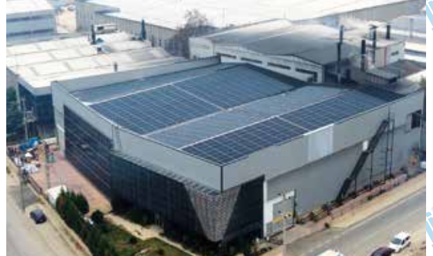
BURSA KESTEL 400 kWp - 2021
